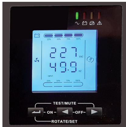
Pannello UPS Rack
